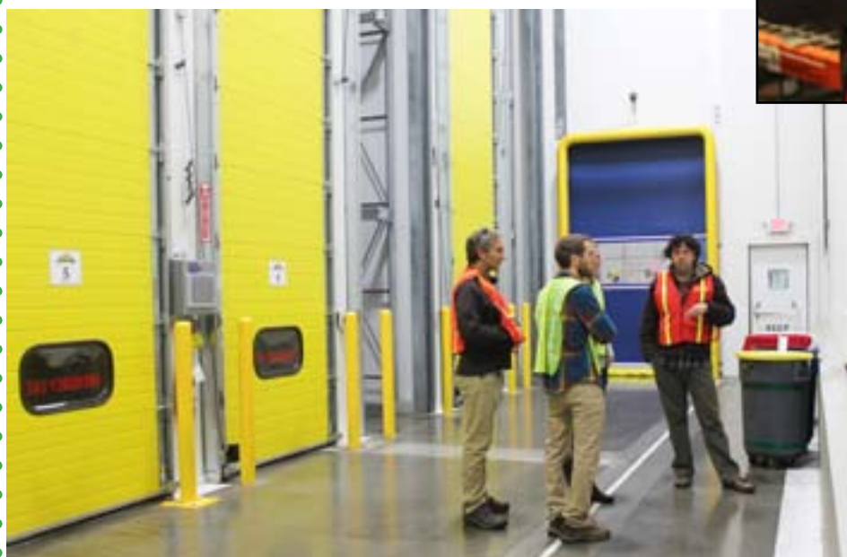
The fruit lockers at left keep bananas at ideal conditions for ripening.
